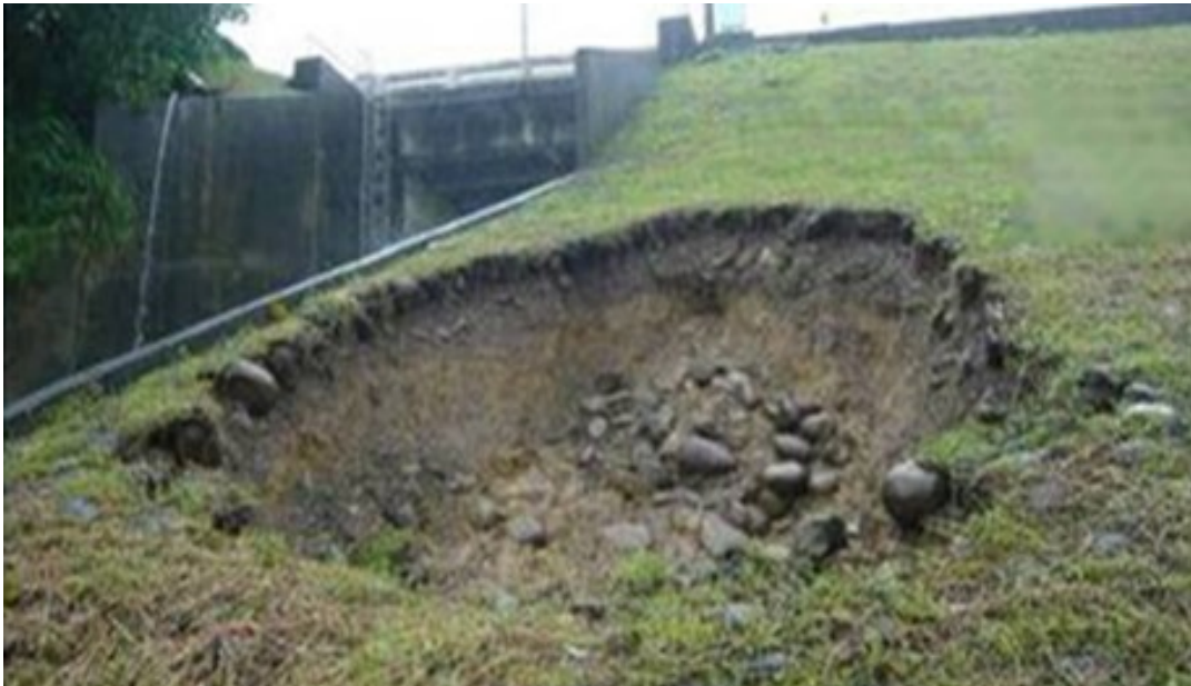
(a) The first sinkhole
