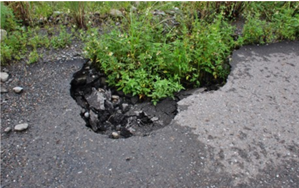
(c) The third road sinkhole
