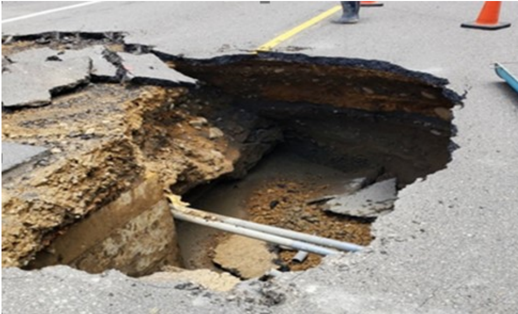
(a) The first road sinkhole
