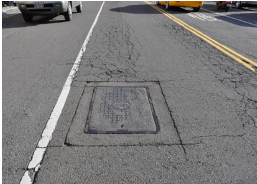
(a) Local cracking
