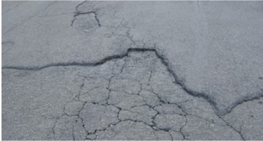
(b) Local cracking and spalling
