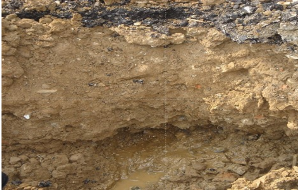
Figure 12. Subgrade soil soaking and softening after rainwater infiltration.
