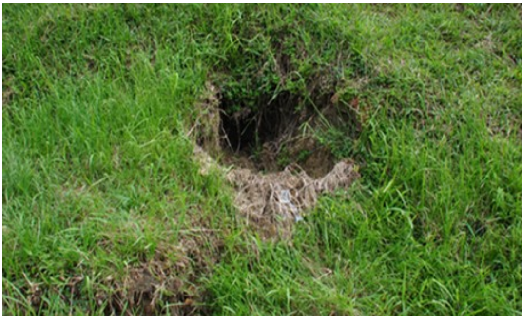
(c) The second and the third sinkholes
