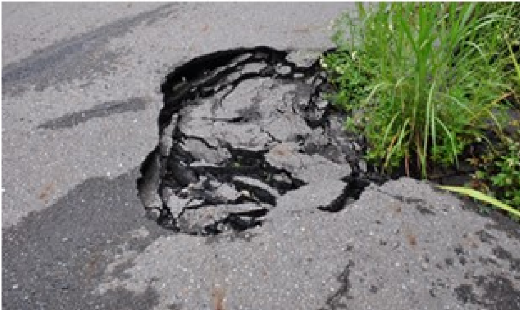
(b) The second road sinkhole
