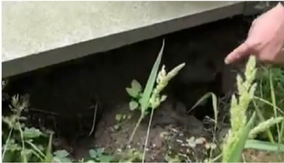
(c) The first community area sinkhole
