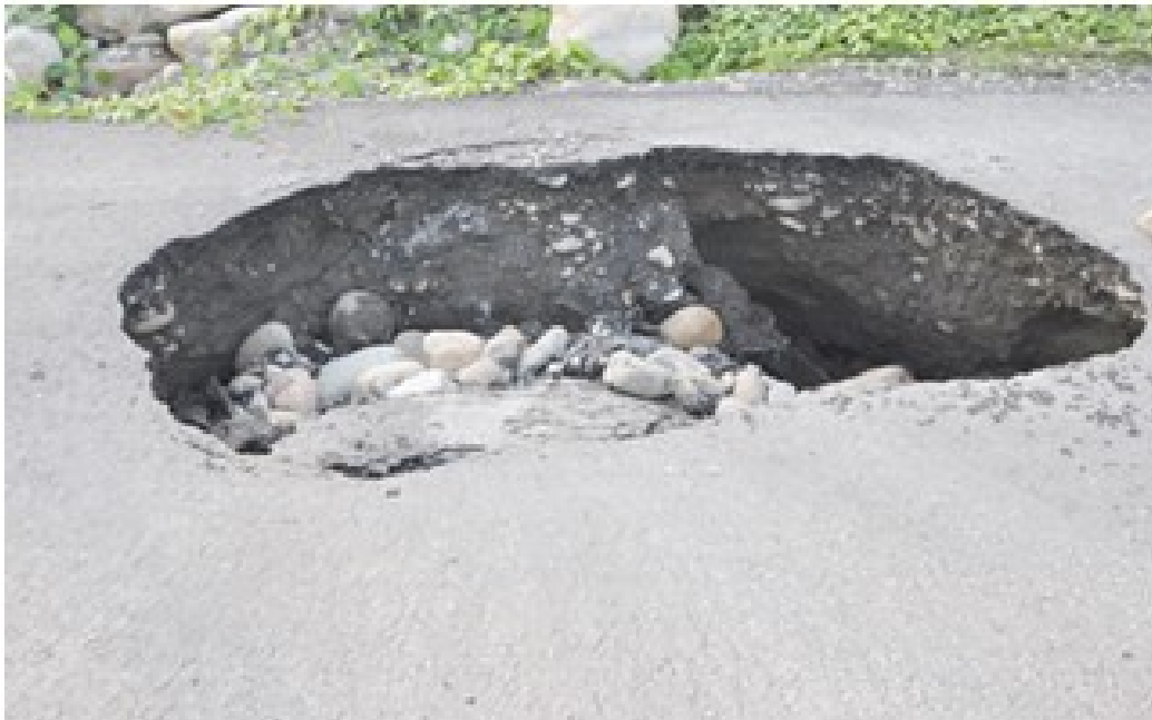
(a) The first road sinkhole
